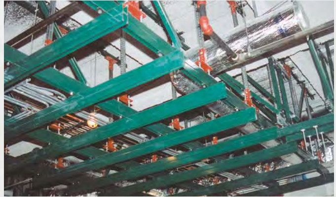
Multi-rail support system with Telespar drops.
